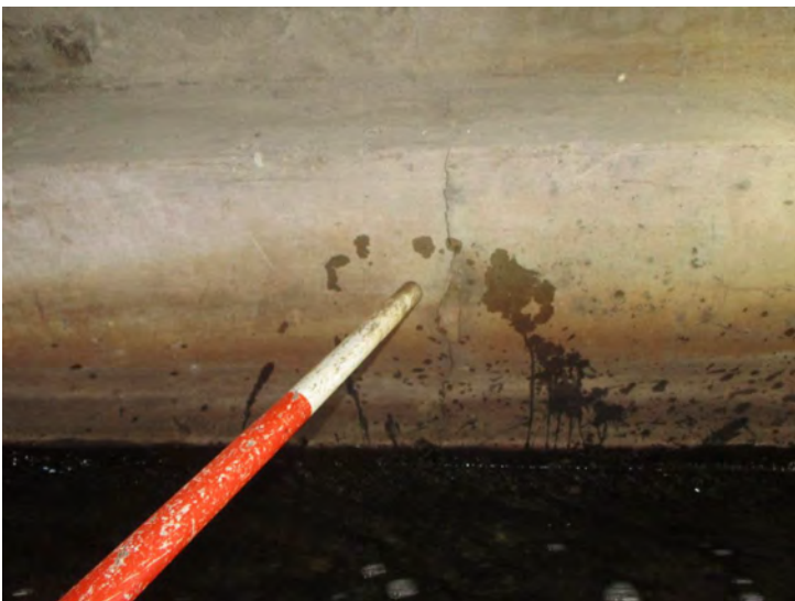
Document Name: 34.JPG Category: Superstructure Span Number: Comments: Span 2w, typical 1/16" cracks in wall
