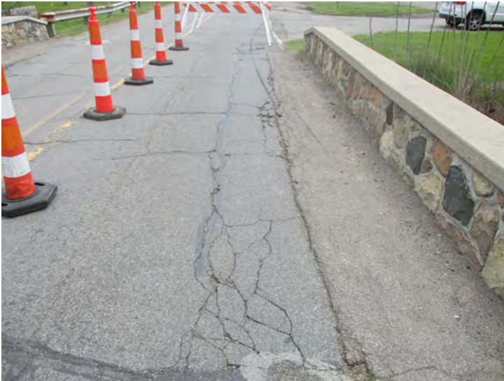
Document Name: 10.JPG Category: Deck Span Number: Comments: Deck surface, eastbound lane, open cracks
