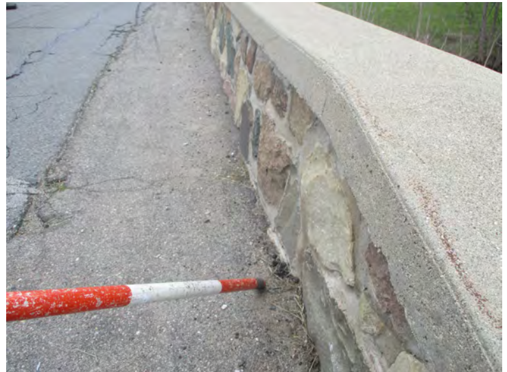
Document Name: 17.JPG Category: Railing Span Number: Comments: South, no separation of railing at impact location.
