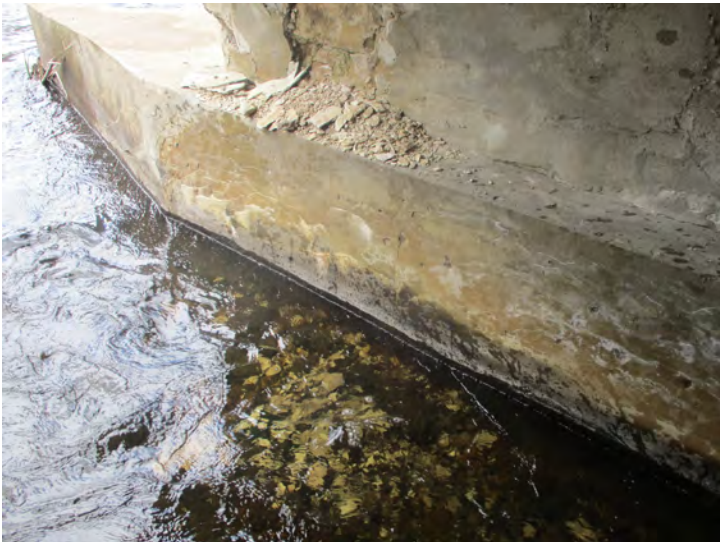
Document Name: 48.JPG Category: Superstructure Span Number: Comments: Span 3w, pier 2w, south end, spall in soffit
