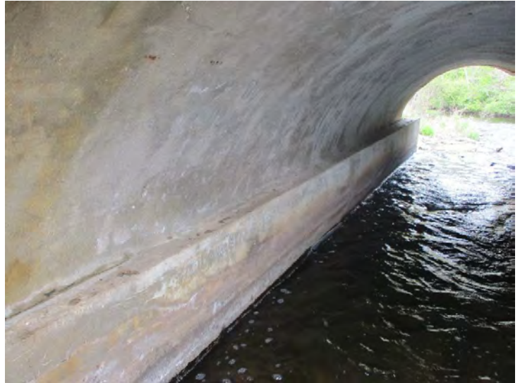
Document Name: 26.JPG Category: Superstructure Span Number: Comments: Span 1w, west abut, looking north
