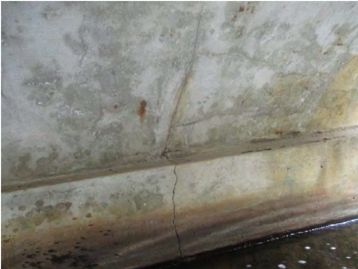
Document Name: 29.JPG Category: Superstructure Span Number: Comments: Span 1w, west abut, 1/8" open crack in wall/footing
