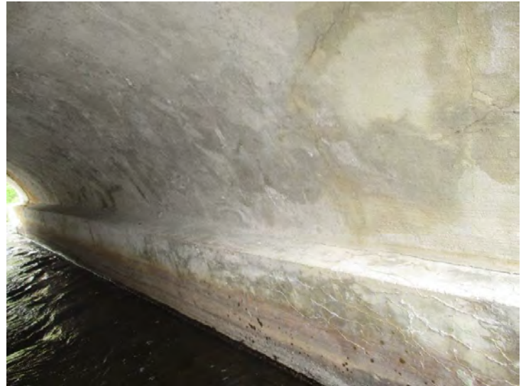
Document Name: 38.JPG Category: Superstructure Span Number: Comments: Span 2w, pier 1w, east face
