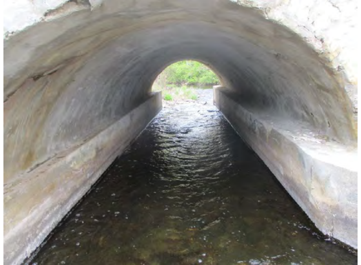
Document Name: 24.JPG Category: Superstructure Span Number: Comments: Span 1w, arch, looking north
