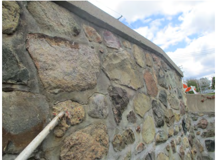
Document Name: 22.JPG Category: Railing Span Number: Comments: South, open crack in mortar in SE
