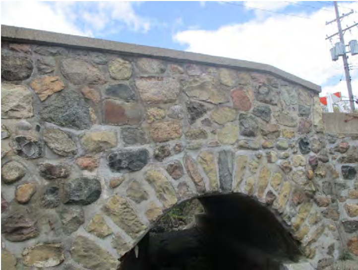
Document Name: 21.JPG Category: Railing Span Number: Comments: South, open crack in mortar in SE
