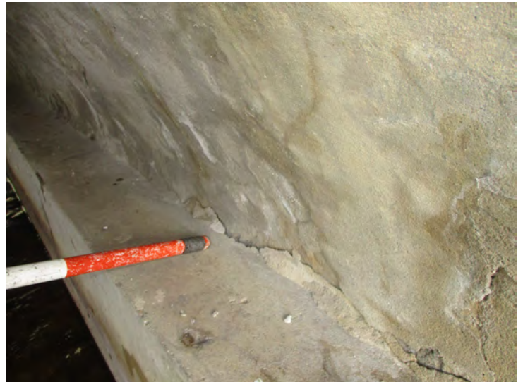
Document Name: 50.JPG Category: Superstructure Span Number: Comments: Span 3w, east abut, south end, 1/8" open crack
