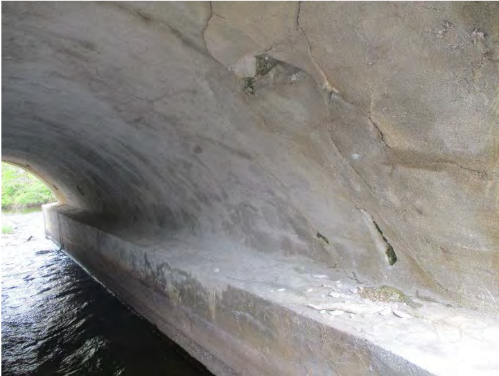
Document Name: 25.JPG Category: Superstructure Span Number: Comments: Span 1w, pier 1w, west face, looking north
