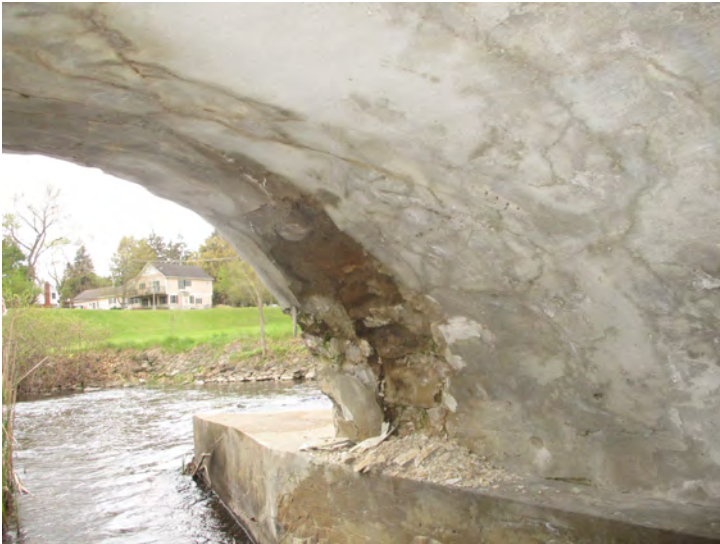
Document Name: 46.JPG Category: Superstructure Span Number: Comments: Span 3w, pier 2w, south end, spall in soffit
