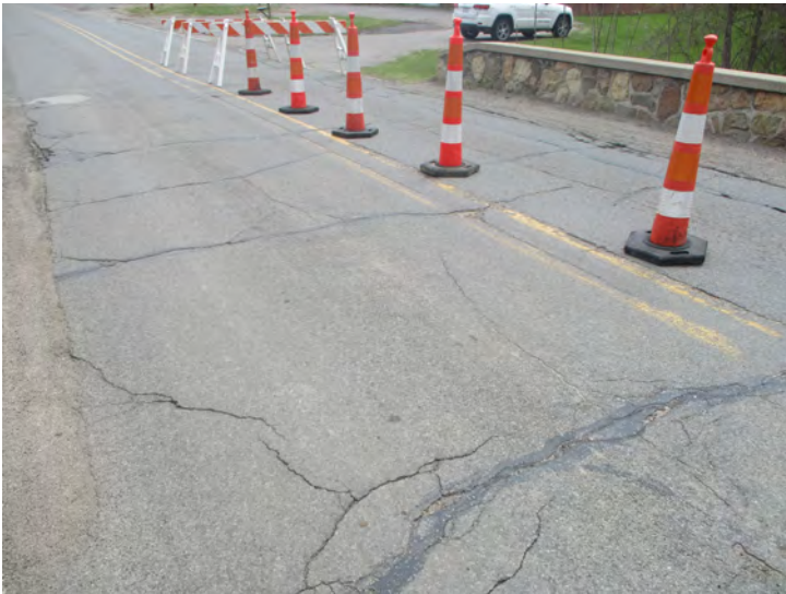
Document Name: 9.JPG Category: Deck Span Number: Comments: HMA surface
