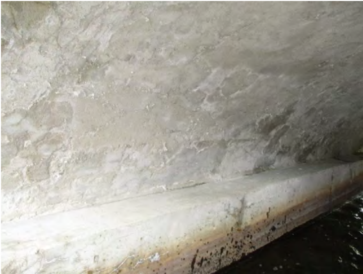
Document Name: 39.JPG Category: Superstructure Span Number: Comments: Span 2w, pier 1w, east face
