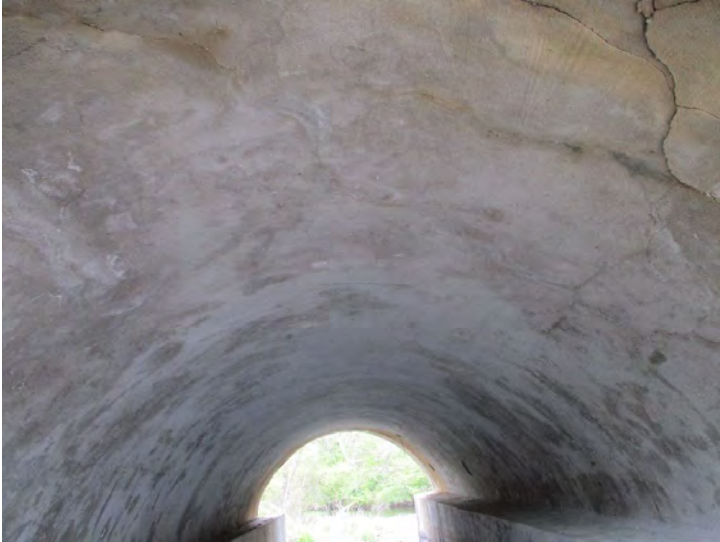
Document Name: 27.JPG Category: Superstructure Span Number: Comments: Span 1w, soffit, looking north
