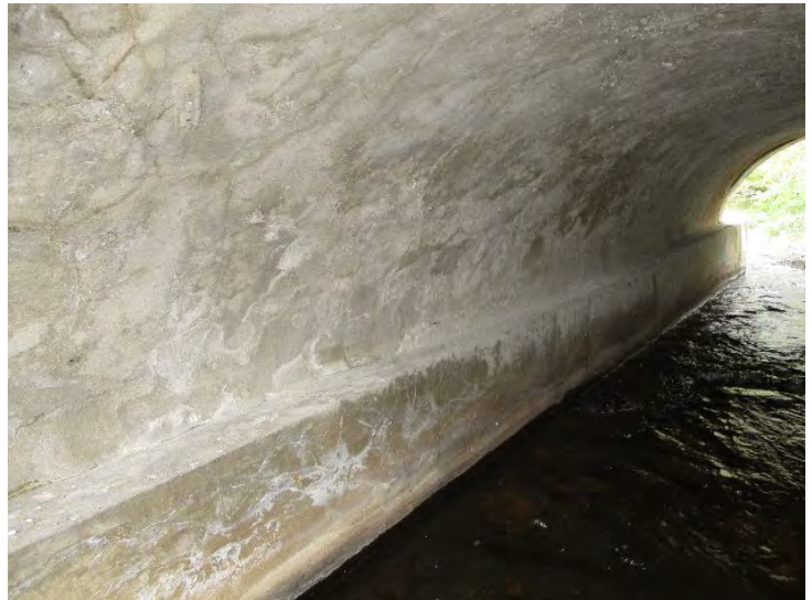
Document Name: 44.JPG Category: Superstructure Span Number: Comments: Span 3w, pier 2w, looking north
