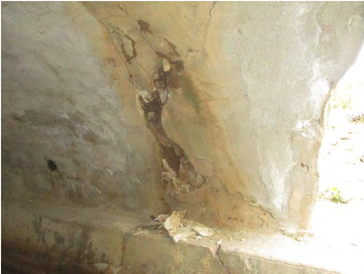
Document Name: 32.JPG Category: Superstructure Span Number: Comments: Span 2w, pier 1w, north end, east face, open spalls/cracking
