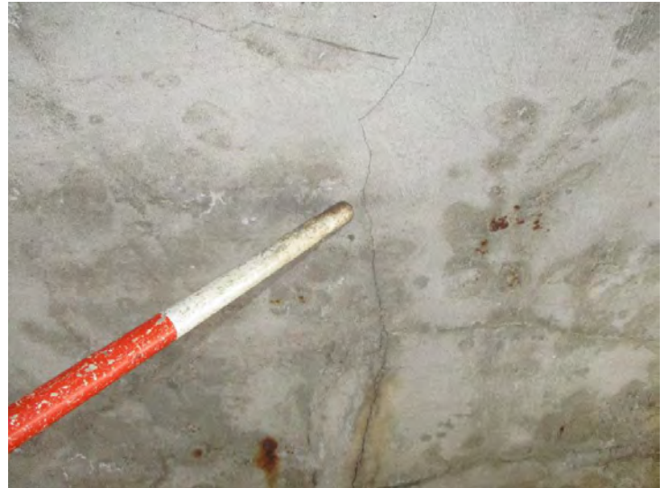
Document Name: 30.JPG Category: Superstructure Span Number: Comments: Typical cracking in arch
