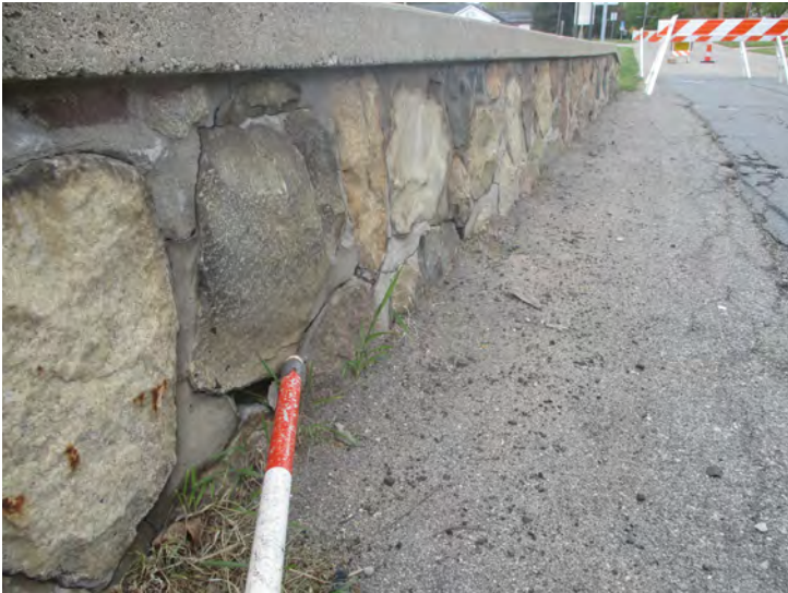
Document Name: 14.JPG Category: Railing Span Number: Comments: South, open cracks in mortar starting in SW
