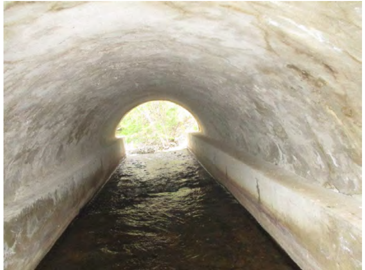
Document Name: 42.JPG Category: Superstructure Span Number: Comments: Span 3w, arch, looking north
