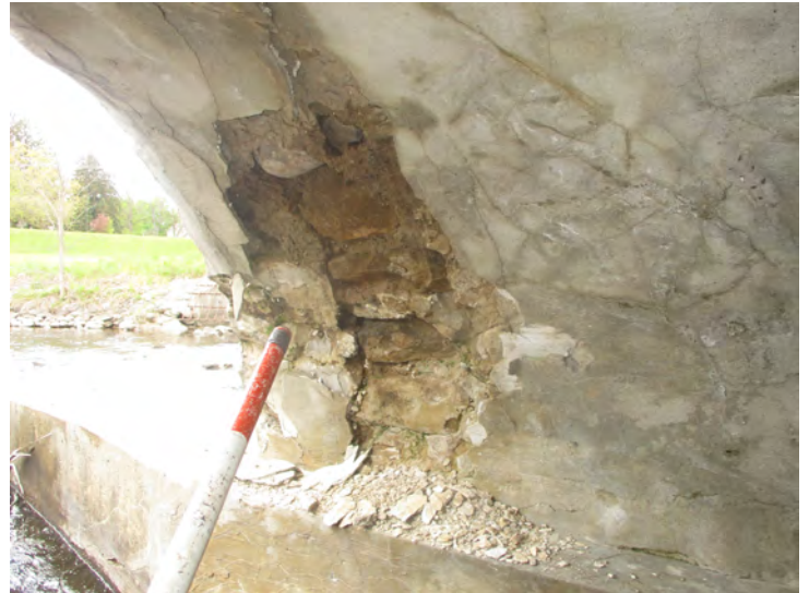
Document Name: 47.JPG Category: Superstructure Span Number: Comments: Span 3w, pier 2w, south end, spall in soffit
