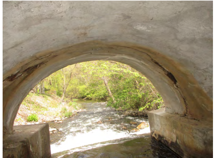
Document Name: 33.JPG Category: Superstructure Span Number: Comments: Span 2w, pier 1w, north end, open spalls/cracking
