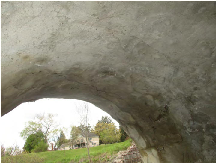
Document Name: 41.JPG Category: Superstructure Span Number: Comments: Span 2w, soffit, south end, open cracks
