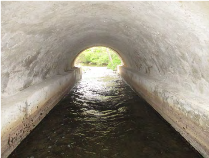
Document Name: 37.JPG Category: Superstructure Span Number: Comments: Span 2w, arch, looking south
