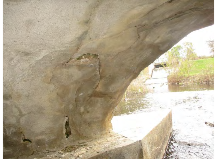
Document Name: 28.JPG Category: Superstructure Span Number: Comments: Span 1w, soffit, SE corner, incipient/spalling with open cracks
