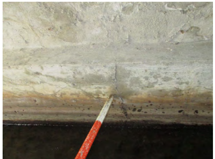
Document Name: 35.JPG Category: Superstructure Span Number: Comments: Span 2w, typical 1/16" cracks in wall
