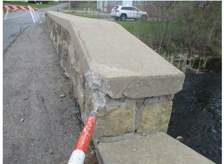
Document Name: 15.JPG Category: Railing Span Number: Comments: South, impact damage in SW
